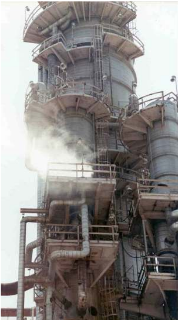
Jet Fuel Leak from Exchanger Joint
