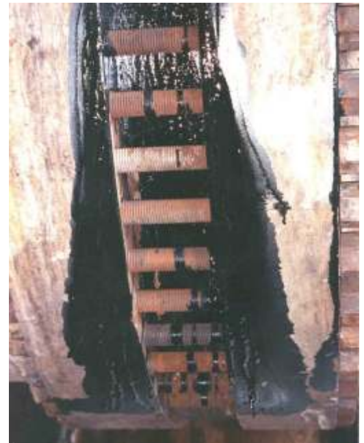
Crude Leak from a Tubesheet
