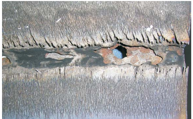
Vacuum Tower Eductor Corrosion
